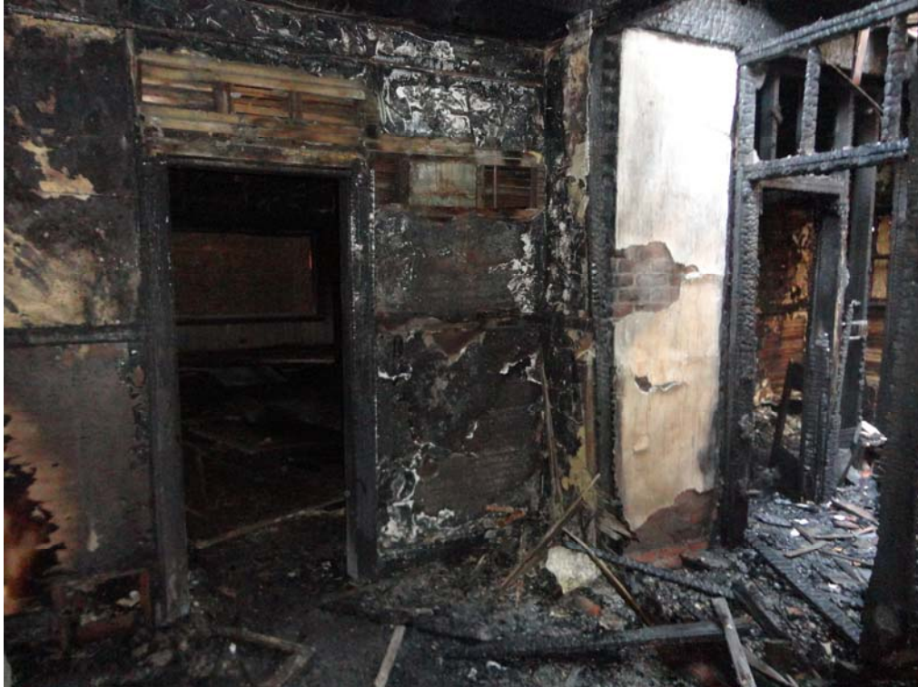
View of the house interior. Fire damage was present throughout limiting access to most of the house.
