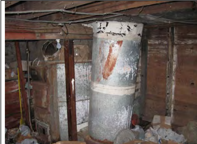
3. Basement: Furnace is on the left hand side; a vertical air duct is on the right hand side. Duct tape (10" strip on top & 4" strip in the middle) is a PACM.
