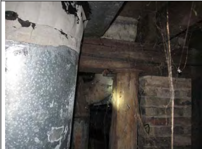
9. Vertical air duct : Duct tape (10" strip on top & 4" strip in the middle is a PACM); Chimney Grout (S-19) is not an ACM.
