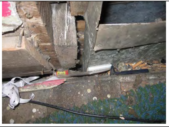
11. Heat register on the 2 nd Floor – no insulation
