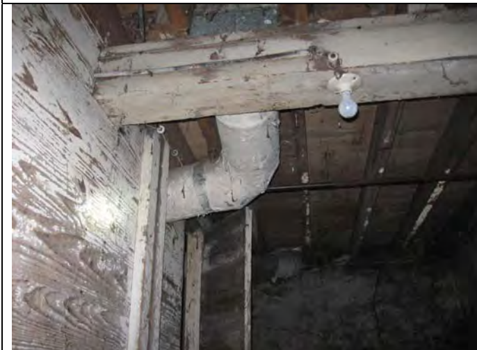
5. Basement: One of the 9"-diameter air ducts that exit the furnace. The ducts are covered in a duct wrap (PACM).
