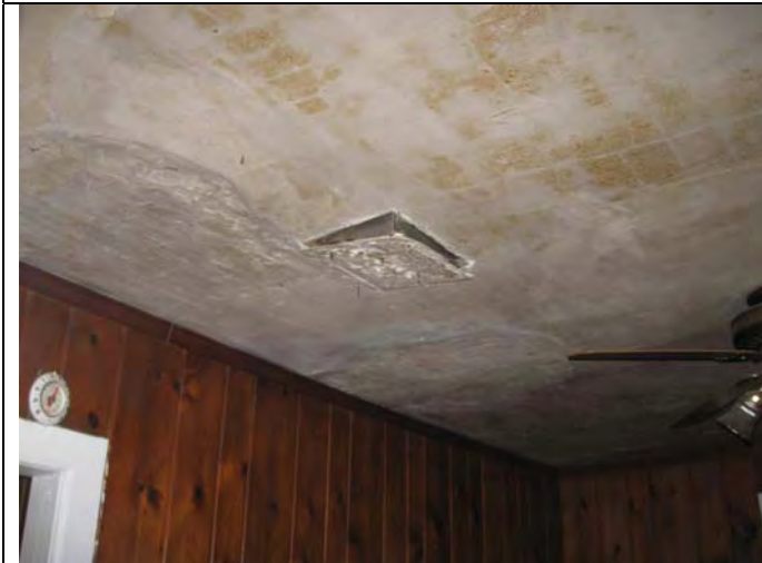
12. Heat register on the 1 st Floor – no insulation. (Note: several registers are covered with flooring and wall board). Wall paper (S-13) covers the plaster (S-12) ceiling (portions).
