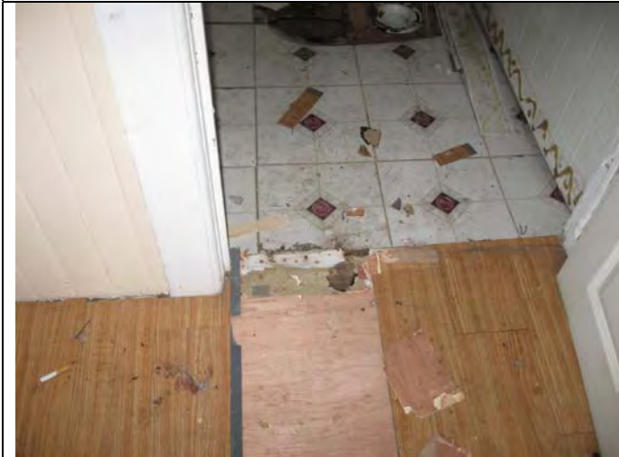
18. 1 st Floor Foyer - linoleum (S-6) and the bathroom (the new 12" x 12" adhesive flooring is not an SACM). The new snap-in surface flooring in the Foyer is not a SACM.
