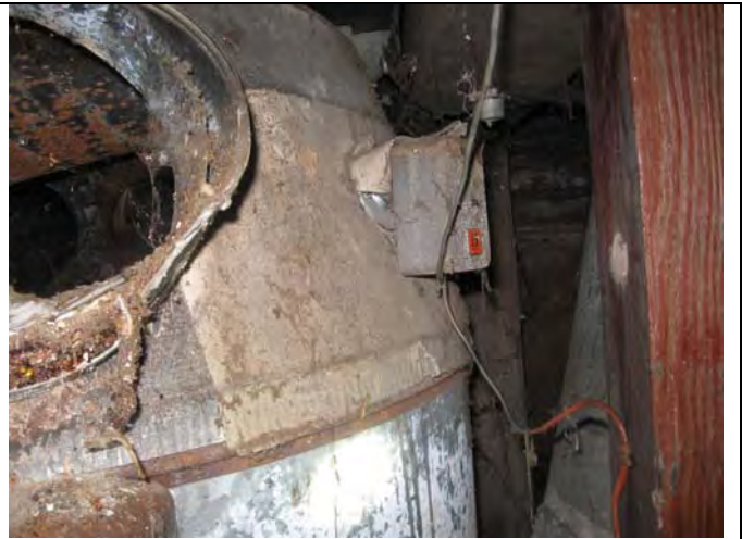
8. Furnace: Note the duct wrap on the furnace and duct "stub" (PACM).
