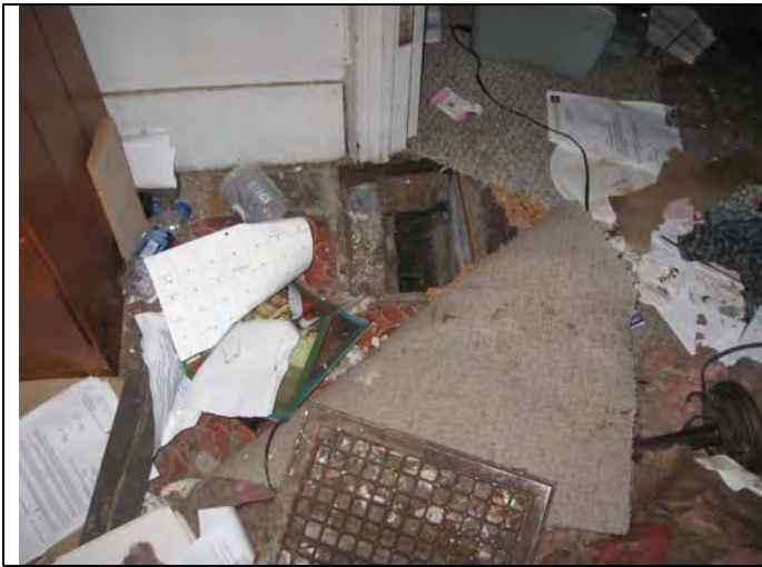
10. Heat register on the 2 nd Floor – no insulation (Note: several registers are covered with flooring and wall board).
