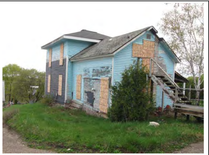
2. Back side view of the house. Note the roofing: S-17 shingles on the front roof; S-18 shingles on the back roof.
