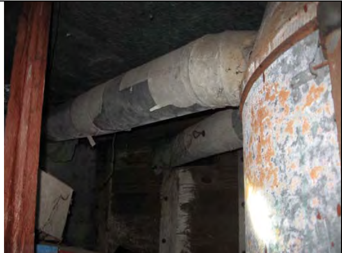
4. Basement: Four, 9"-diameter air ducts exit the furnace. The ducts are covered in a duct wrap (PACM).
