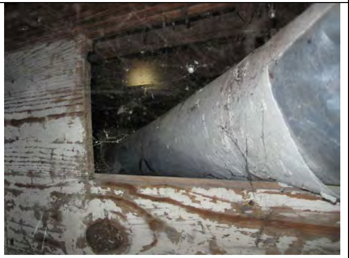
6. Basement: One of the 9"-diameter air ducts that exit the furnace. The ducts are covered in a duct wrap (PACM).
