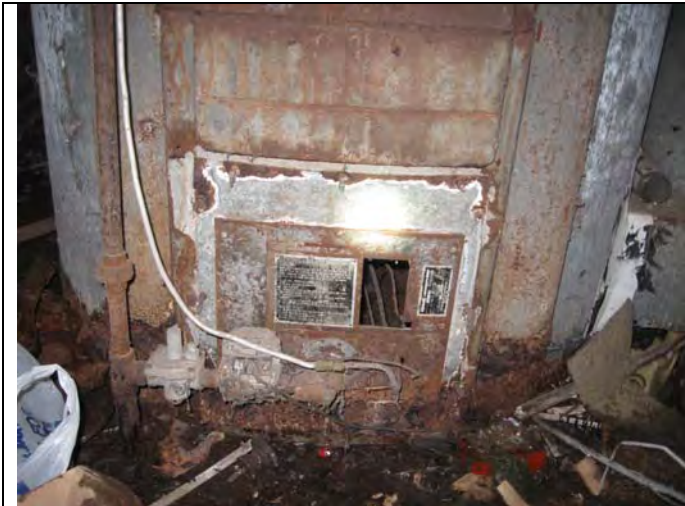
7. Furnace: The gasket/seal around the access door is a PACM.
